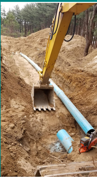
Photo: Installation of underground piping connecting groundwater extraction wells to a PFAS treatment system at BNL.
